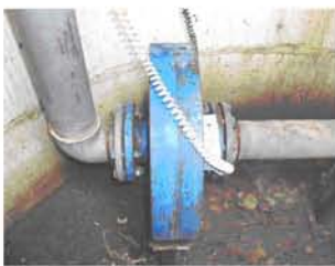
The Hydromag installed in Osterby's main drinking water distribution shaft
