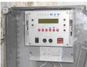
The integral control box mounted in an additional protective casing
